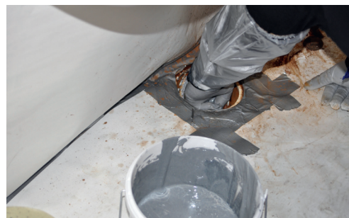
2. The coating is spread by hand onto the surface of the floor drain.
